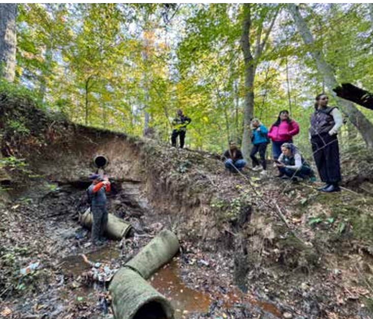
This exposed culvert is just one example of the impacts resulting from channel instability.
